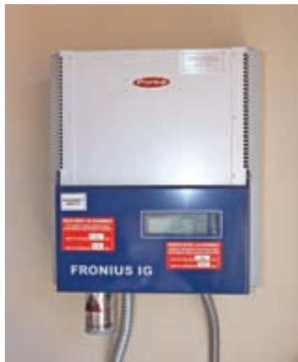
Grid-direct inverters allow PV systems to be simpler, less expensive, and, therefore, more cost-effective than their battery-based counterparts—but PV systems still need significant cost decreases to catch up with the high efficiency of SHW systems.
