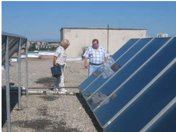
Figure 2. General view of the solar collectors.
